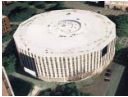
In addition to it's functional and social problems, Harrelson Hall, NCSU, also has foundation problems and is sinking.
