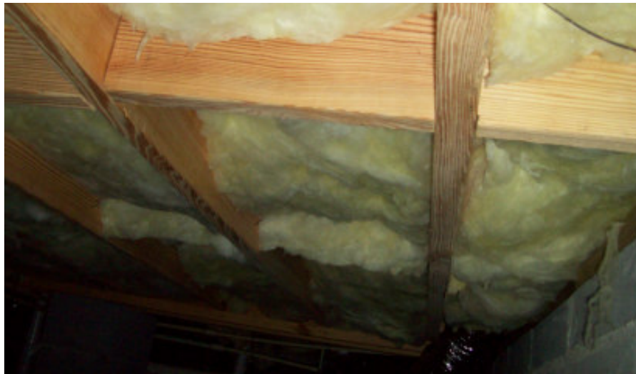
Batt insulation without vapor barrier will fail.
